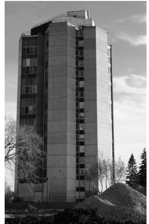
After years standing tall at the centre of Michener Park, Vanier Tower is being demolished in advance of site redevelopment. (PHOTO: Mike Kendrick)
